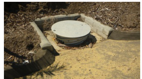
Fig. 9. Drainage inlet surrounded by concrete berms. Water enters inlet from an adjacent asphalt road which is located at a low point on the property. Flow velocity of the water slows down prior to entering inlet, allowing sediment to drop out of the water. After entering the inlet, corrugated plastic pipes convey water underground. Photo: S. Webb, courtesy of the Resource Conservation District, Ventura County.
